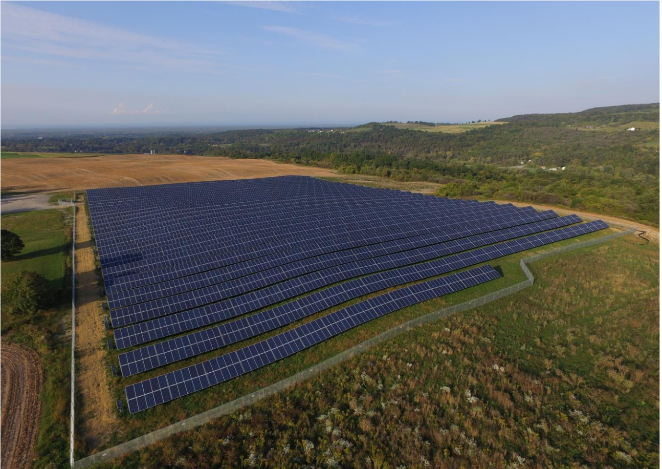
Madison County 2.4 MW Solar Array
